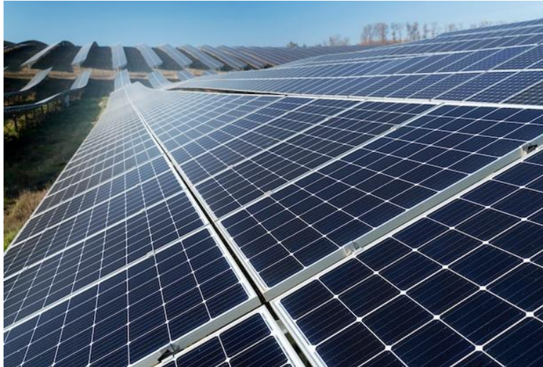
Location: Aruppukottai Total Capacity – 2 MW
